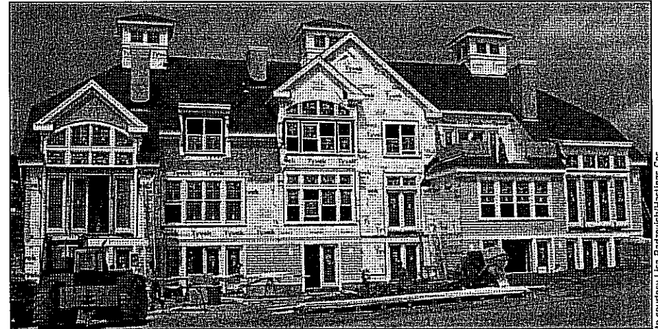
The BackRiver Townhomes luxury condominium development is being built at 224 Beal St. in Hingham.
